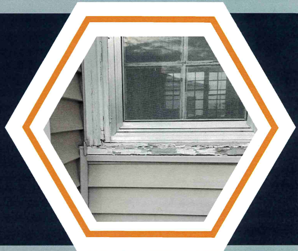
Picture of TRPHD's first lead assessment in the district. This paint is positive for lead. This house is in Dawson County.
